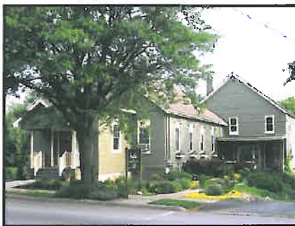
Along with the tower went rotting sills and constant water problems.
